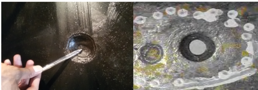
Microbiological Induced Corrosion
